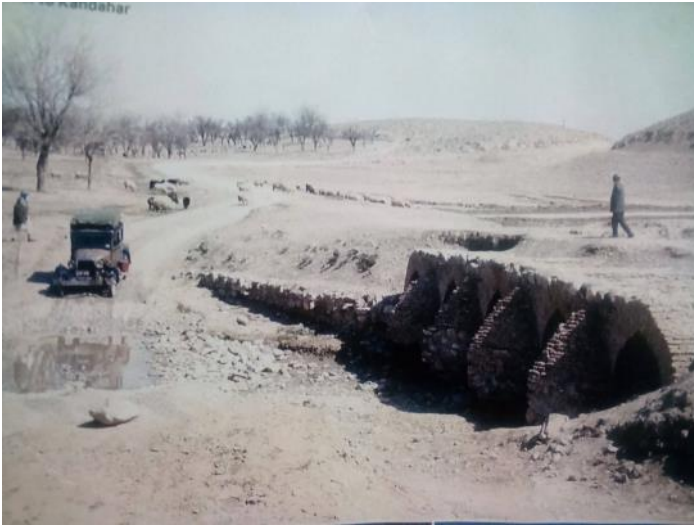
One of 83 washed out bridges on the road from Kabul to Kandahar in Afghanistan.
